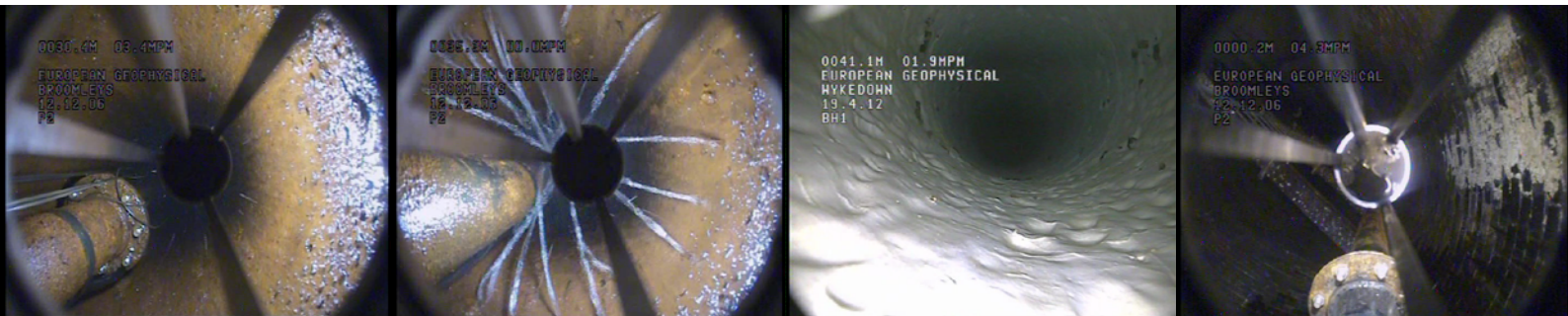
Rising main join in 600mm id plain steel lined borehole
